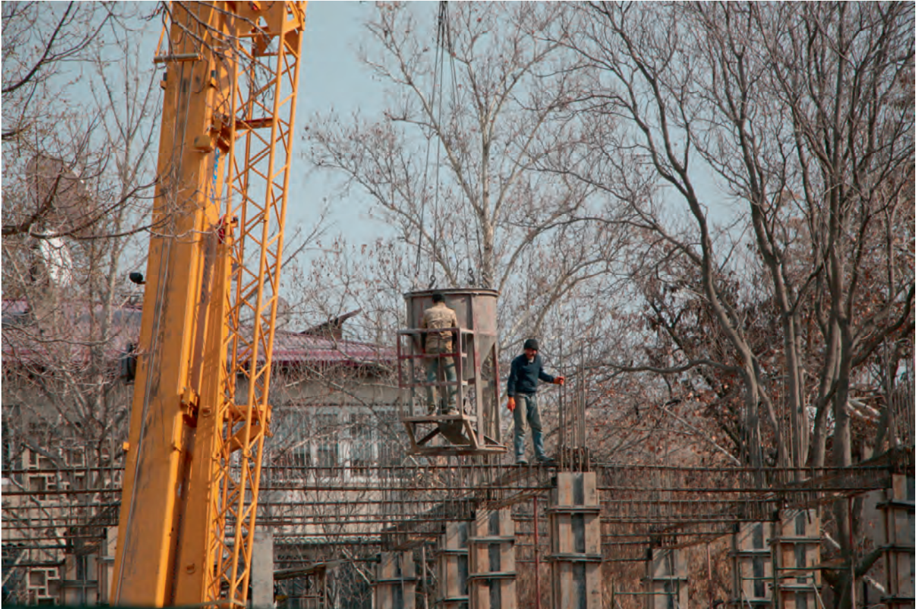
Photo 16.1: Construction of a multi-storey car park in the centre of Tashkent City
