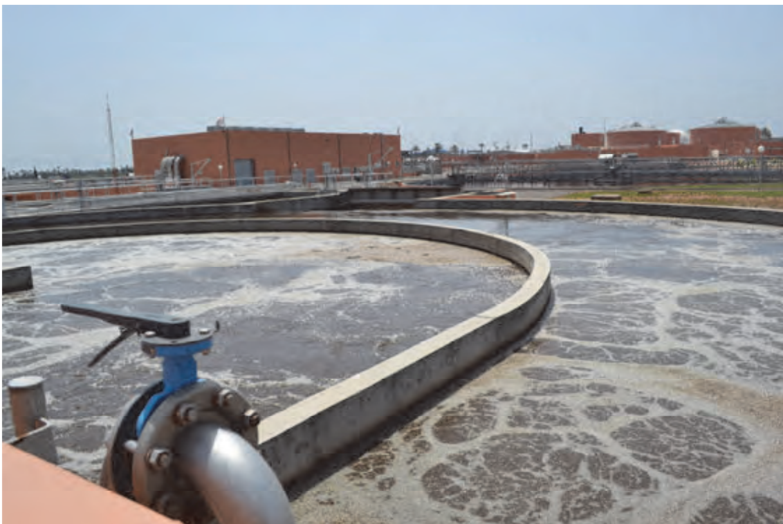
Photo 9.5: Marrakech wastewater treatment plant
